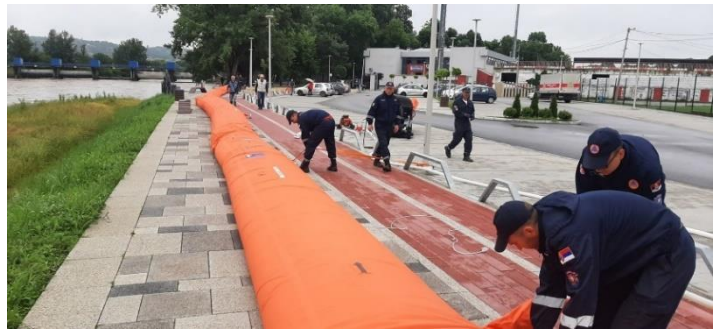
Picture 3 - Setting up mobile dams to protect the critical infrastructure in the City of Cacak, June 2023
